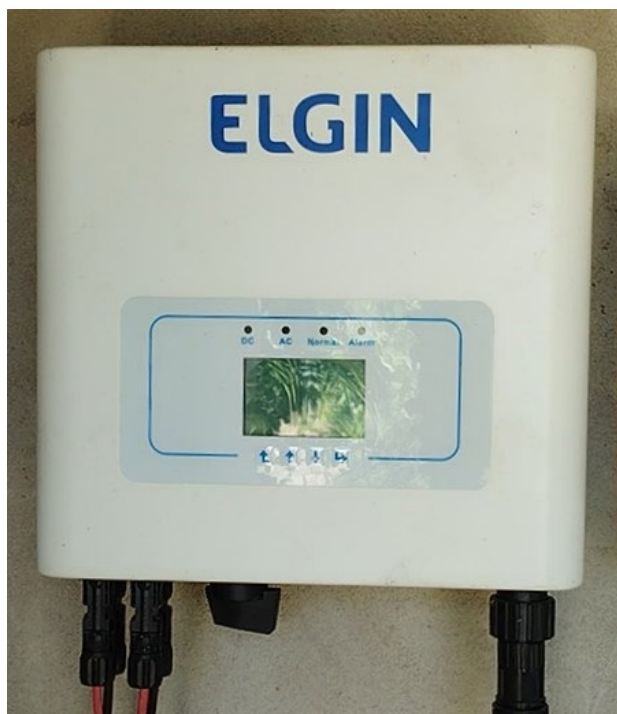
Figura 16 – Inversor solar On-grid
